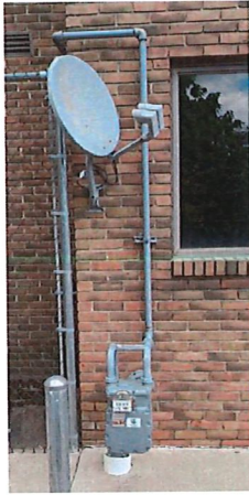
GAS ENTRY WITH METER AND REGULATOR
