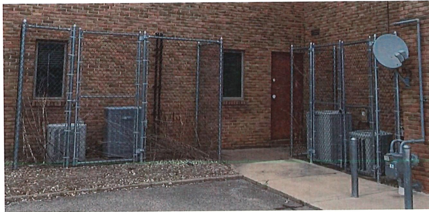
CONDENSING UNITS ON SOUTH SIDE
