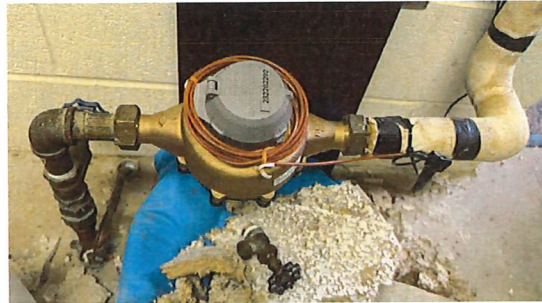
WATER ENTRY AND METER
