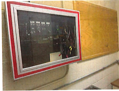
EXISTING FIRE ALARM SYSTEM
